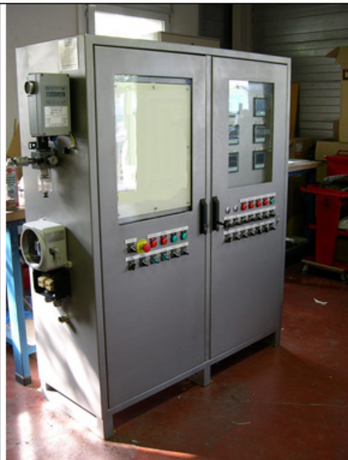
double door cabinet for process management
