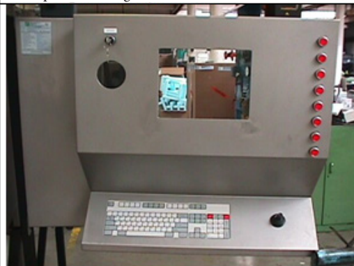
pc cabinet process management
